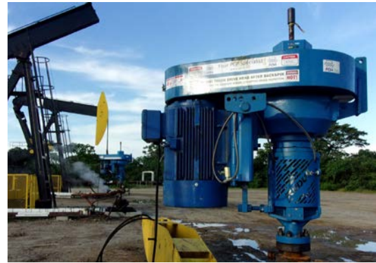
Figure 14: Well B Drivehead (Well A at the back)
